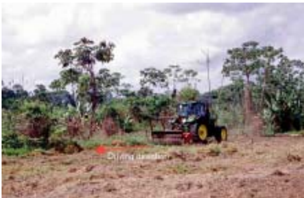
Burning the fallow vegetation destroys all the biomass accumulated during the fallow period. The tractor mounted bush shredder is an alternative. It cuts the bush vegetation into small pieces, thus producing a mulch layer. The subsequent crop is planted directly through the mulch. (Photo: M. Denich)
